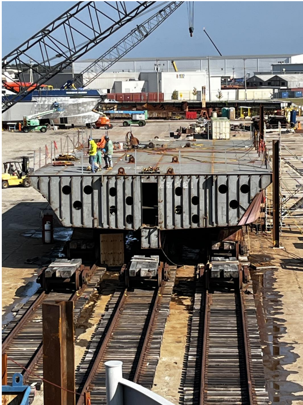
3264 – View of Portion of Shipyard and the first three modules being assembled. Working on deck welds.
