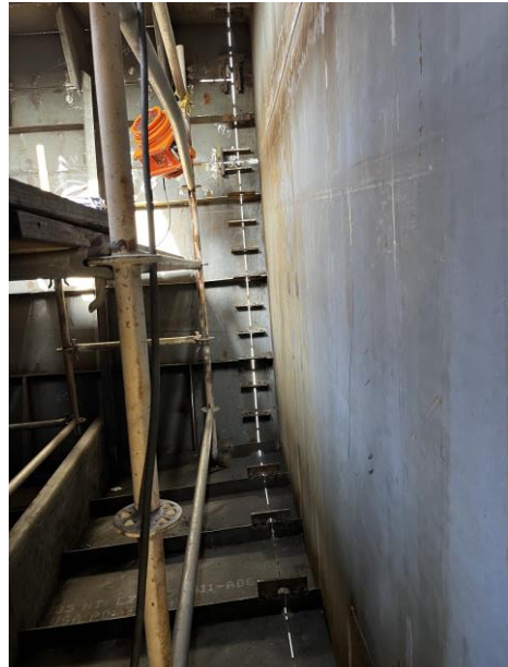
3087 – Strong Backs on the Master Butt between 3 & 4. These help hold the seam at the proper alignment
