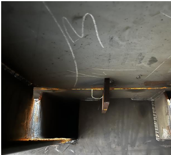
3223 – Master Butt Joint for Modules 3 & 4. Note the strongback plate holding joint in alignment.
