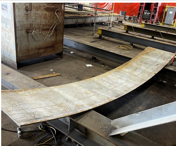
3146 - Guard plate after coming out of the break press. Conforms the plate to the curve of the vessel.
