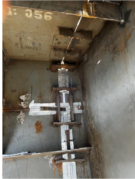
3227 – Preparation of Master Butt Joint so can weld from outside. Ceramic tape is used to help properly contain weld.
