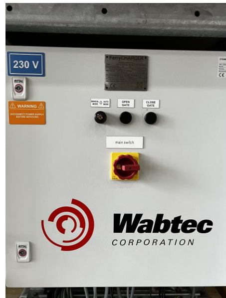
3261 – Control Panel on socket
