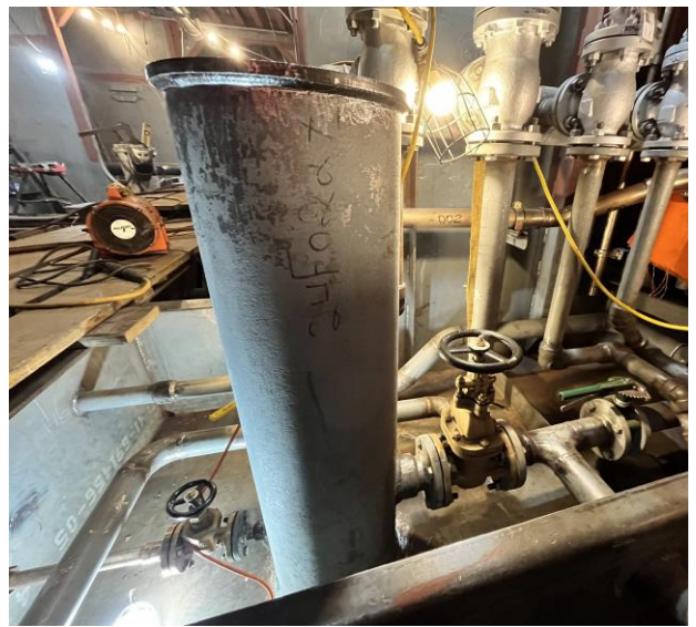
5102 – Seachest (Draws in sea water for keel coolers and sprinkler system)
