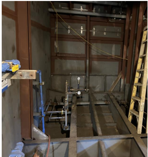
2596 – Generator Space with Fuel Lines
