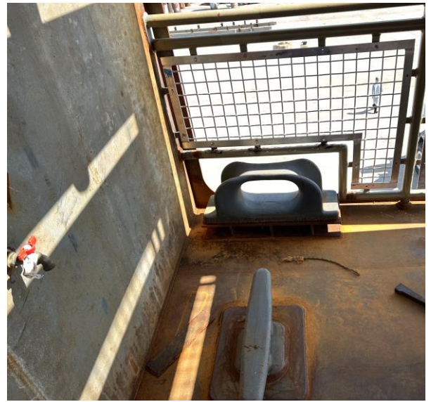
2603 – Cleat w/Line Chock at Handrail Penetration
