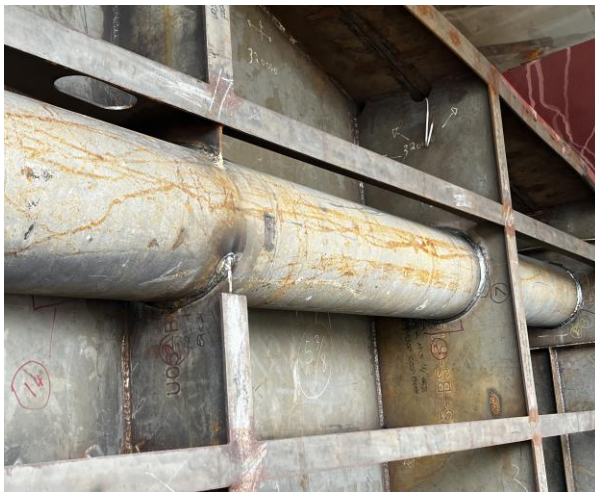
4894 – Welding up Stern Tube (This is a slow process due to expansion of steel during welding and the need to maintain very tight alignment dimensions. Welding is very sequential to control alignment movement)
