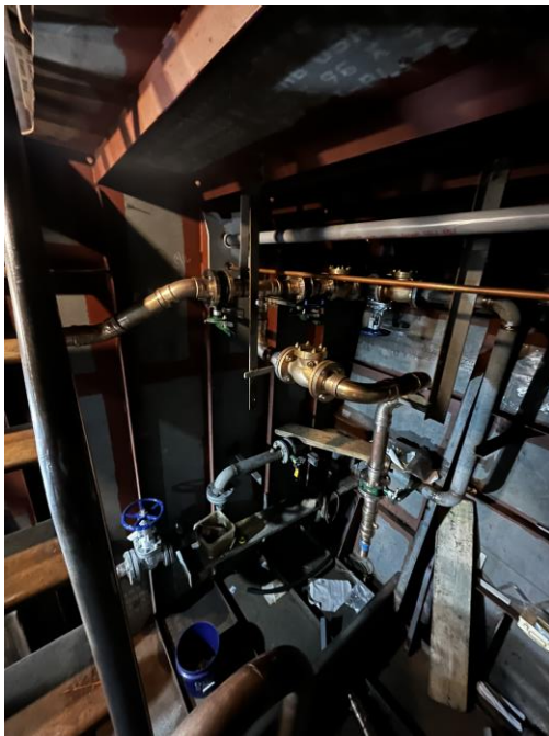
4850 – Fire Main Valves
