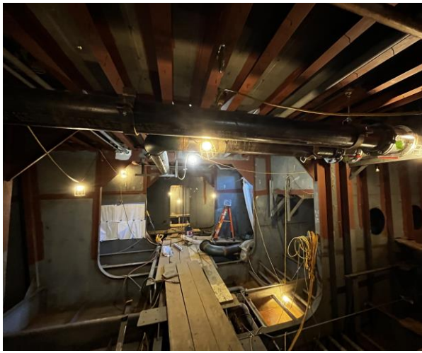
4841 – General View of the Engine Room
