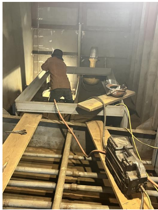
5042 – Support Frame for Sanitary Sewer Tank
