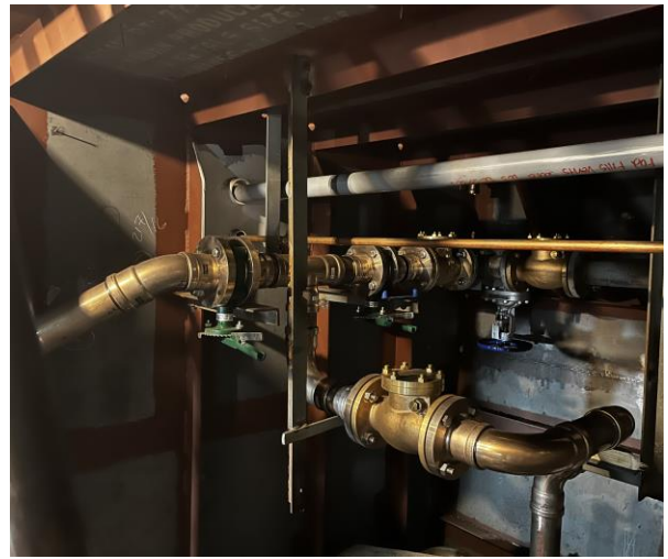
4848 – Fire Main Valves & Fittings
