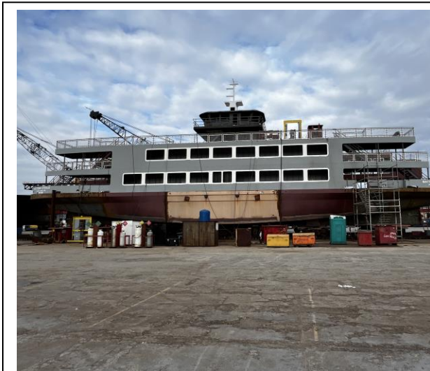
4955 – Paint Prepping Around Windows for Window Installation (Note that the handrail sections are in place with screening)
