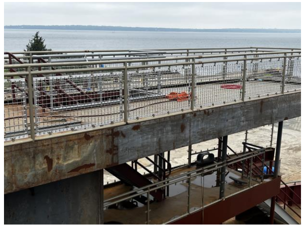
4898 – Railing with and without screening
