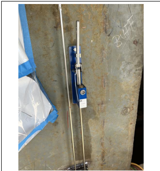
5008 – Emergency Fuel Shutoff
