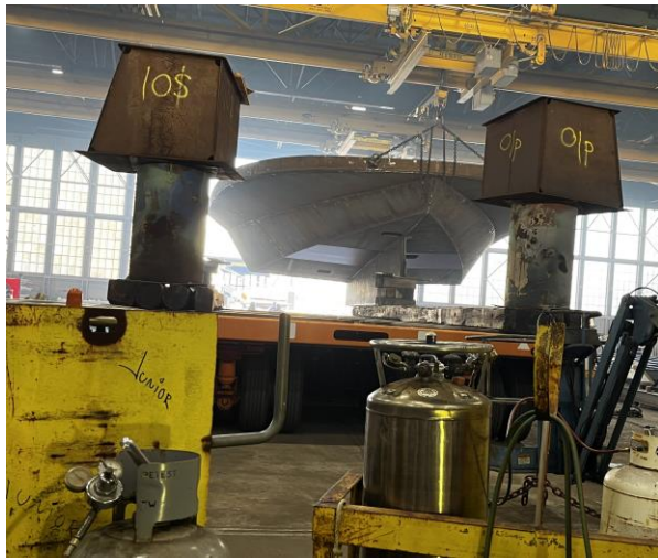
3438 – Module 5 Being Loaded onto the Trailer to be Moved to the Assembly Area
