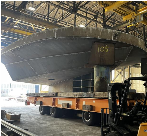
3347 - Module 1 Lifted and Ready to be Loaded on Trailer, Trailer Almost in Place Under the Module
