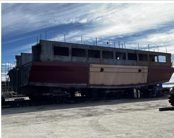
3330 - All Module 7 Longitudinal Bulkheads in Place for the Main Deck Cabins. 01 Deck Plate in Place over Starboard Cabin.
