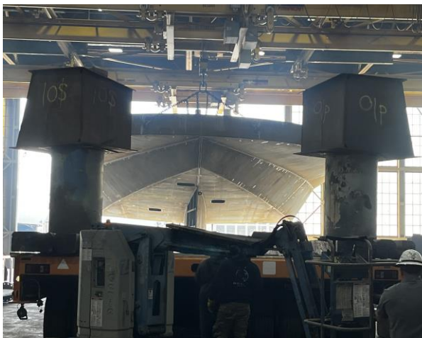
3345 - Module 1 Lifted and Ready to be Loaded on Trailer, Moving Trailer Under the Module
