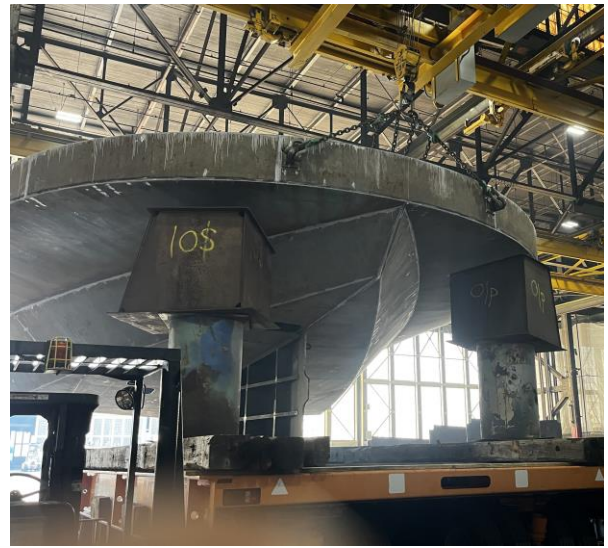
3348 - Module 1 Lifted and Ready to be Loaded on Trailer, Trailer Almost in Place Under the Module
