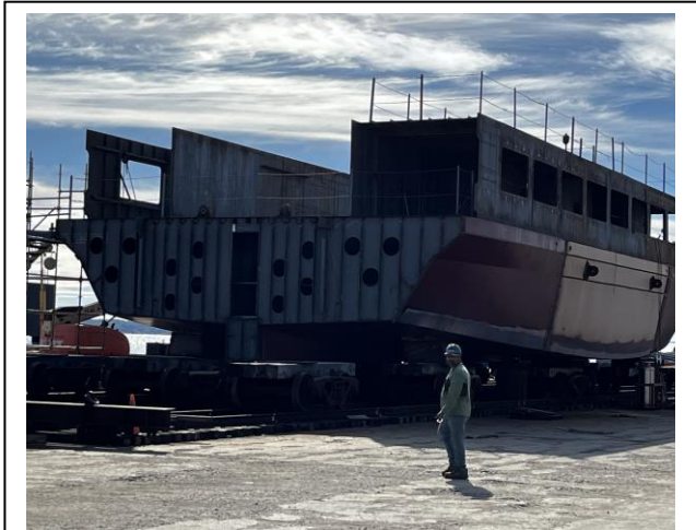
3329 – All Module 7 Longitudinal Bulkheads in Place for the Main Deck Cabins. 01 Deck Plate in Place over Starboard Cabin.
