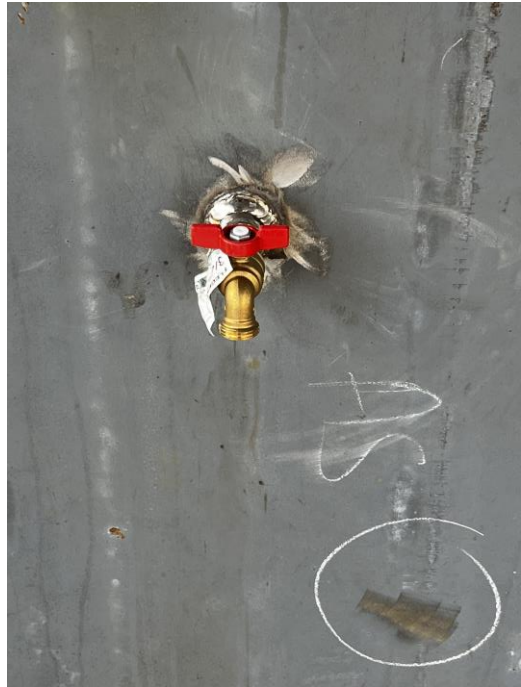
4347 – Potable Water Spicket – Main Deck
