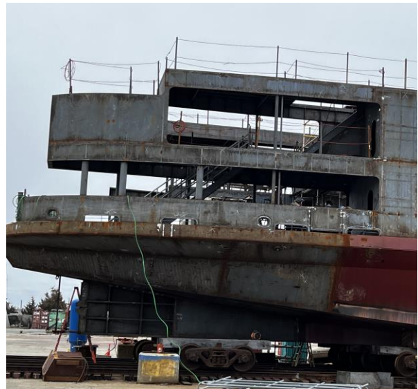
4164 – Starboard Stern w/Charger Socket Box in Place (left side of picture)
