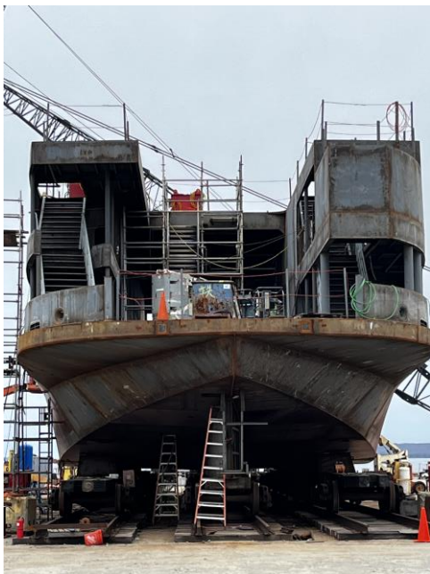
4163 – View of Stern End w/Charger Socket Box in Place (right side of picture)
