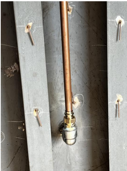
4348 – Potable Water Piping
