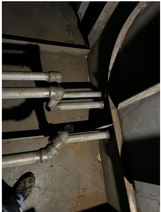
4505 – Piping in Engine Room
