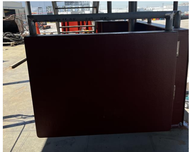
4487 – Typical Swing Gate at Man Overboard Station
