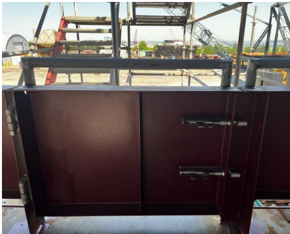
4485 – Typical Swing Gate at Man Overboard Station
