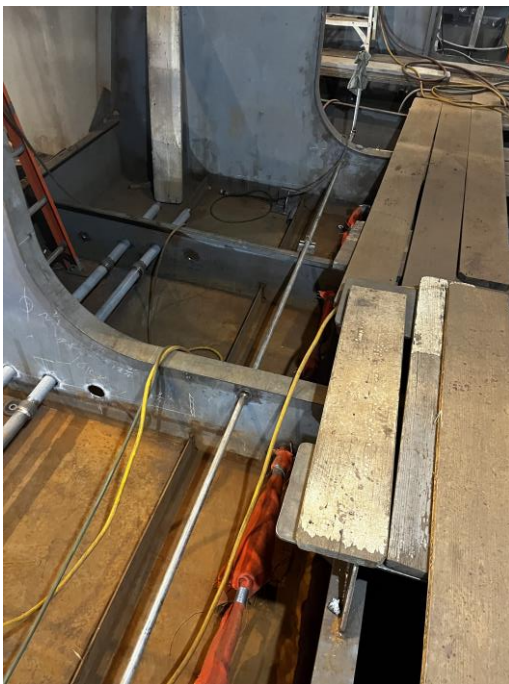
4506 – Piping in Engine Room
