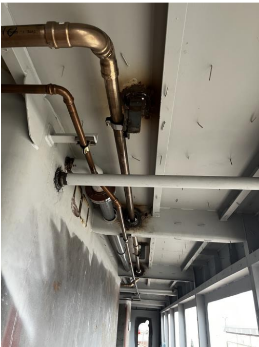
4764 – Piping in 01 Deck Starboard Cabin
