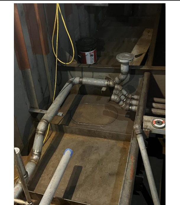
4688 – Piping Manifold Area
