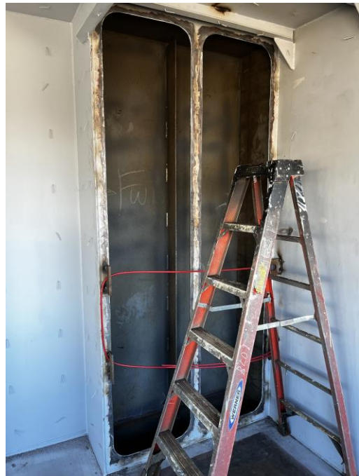
4570 – Systems Chase on 01 Deck
