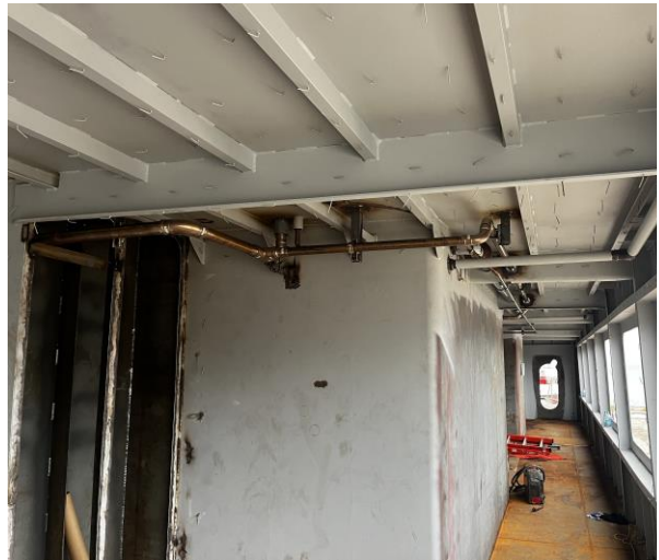
4763 – Piping in 01 Deck Starboard Cabin
