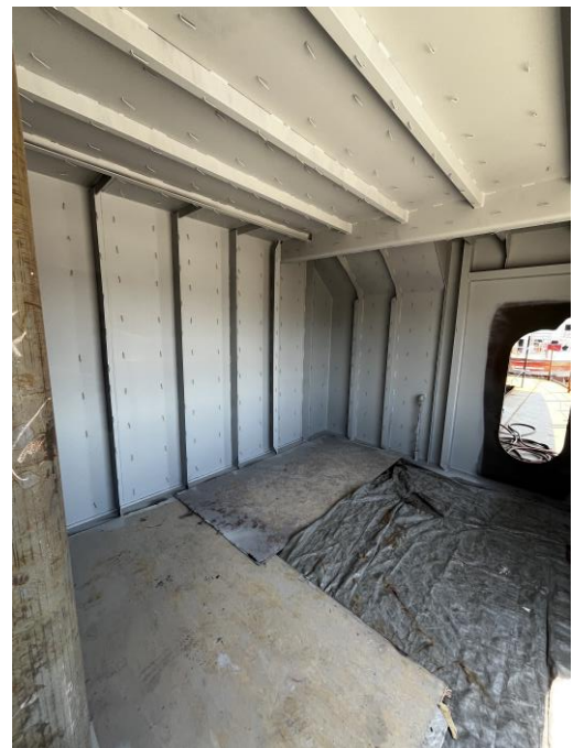
4507 – Paint Coat in Main Deck Starboard Cabin
